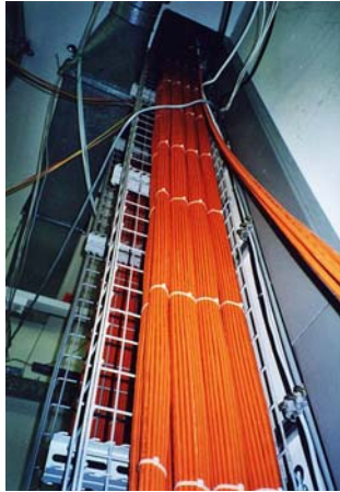
Figure 3. Alien NEXT becomes a critical factor when a lot of unshielded cables run parallel to each other over long distances, as in this riser zone.
